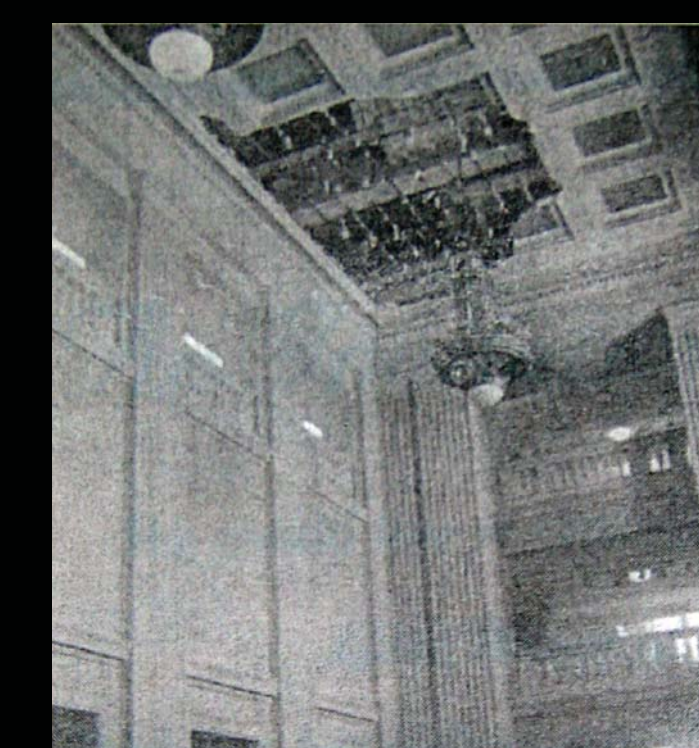
Figure 7: Part of the ceiling in Memorial Hall collapsed in 2001.
